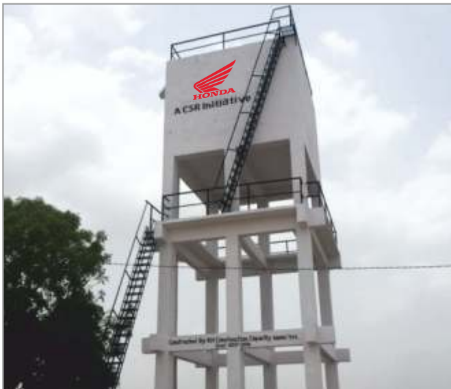
Overhead Water Tank - capacity 50,000 ltr.
