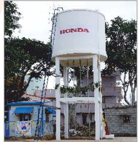
Overhead water tank 50,000 Ltr. at Karinyakanhalli, Karnataka
