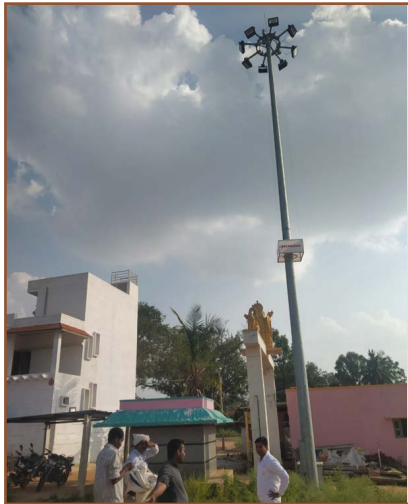
High mast street lights installed
